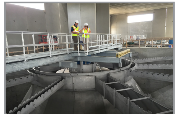
One of three solids contact units at the new Water Treatment Plant.
