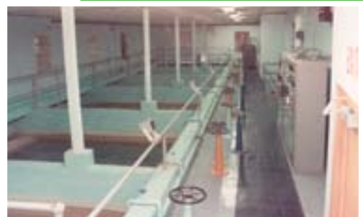
Water Treatment Plant Filter Room (1989)
