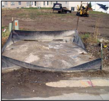
This washout needs to be maintained and is too close to the street.
