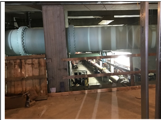
View into the lower pipe gallery from a first floor observation window.
