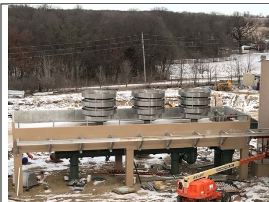
Cascade Aerators, viewed looking north towards E. 13 th Street.
