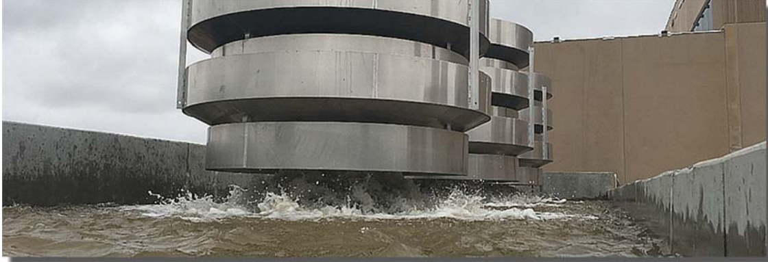
Stainless steel "cascade-style" aerators at the new Water Treatment Plant during a raw water high flow test on April 27.
