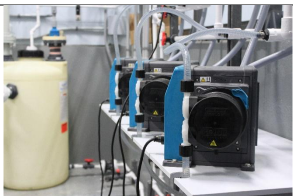
Chemical feed pumps installed and ready
