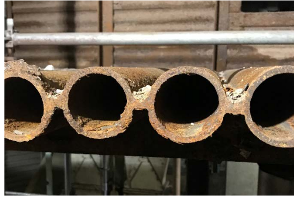
Figure 3 Bottom Tubes on Rear Wall
