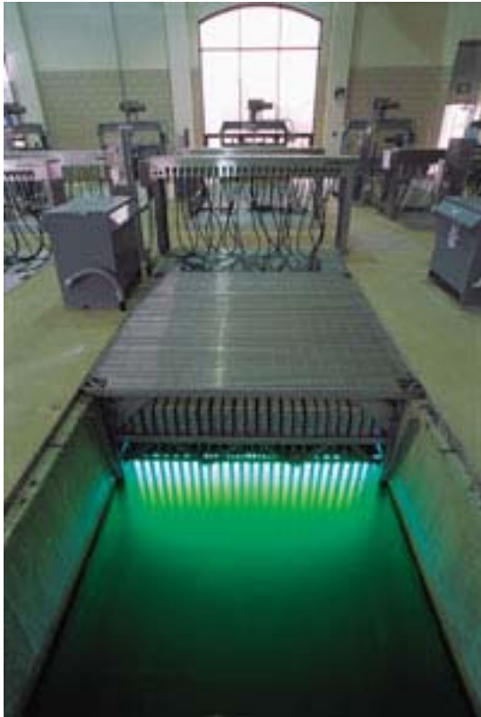
Vertical UV Disinfection Setup
