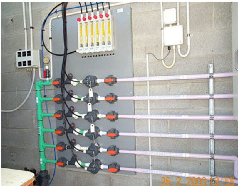
Chlorine Injection Network
