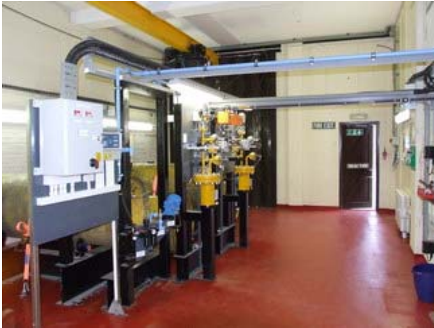
Chlorine Gas Dosing
