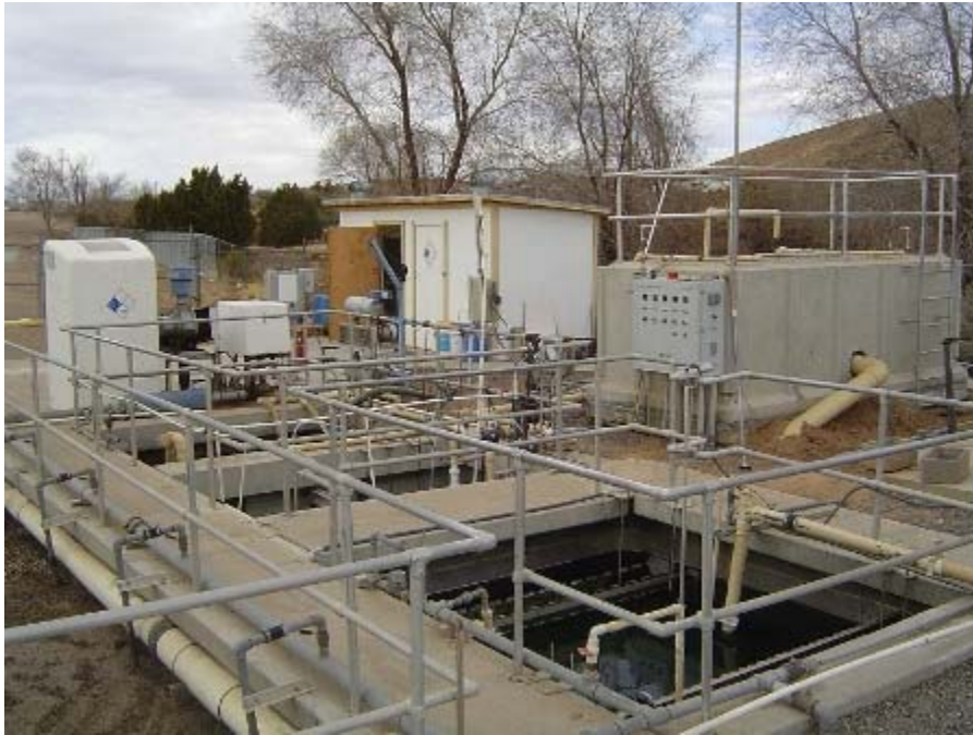
Ozone Disinfection at a Wastewater Plant
