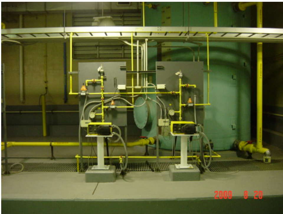
Sodium Hypochlorite Storage and Feed System – Omaha WWTP
