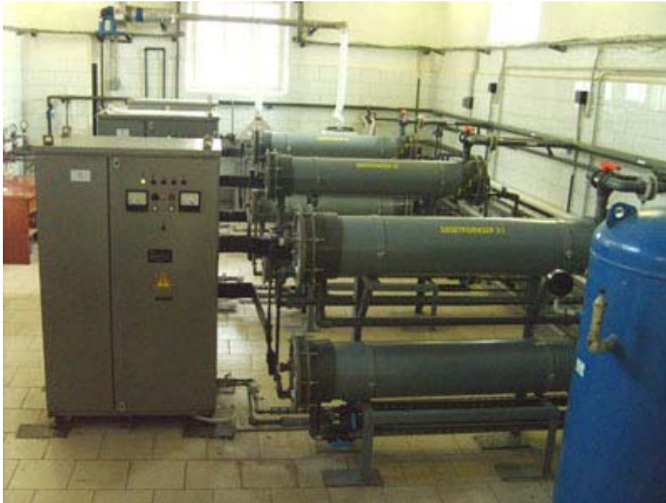
Sodium Hypochlorite Generation
