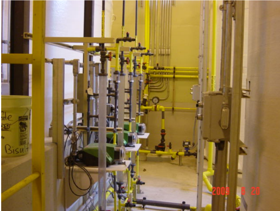
Sodium Bisulfate Storage and Feed System – Omaha WWTP
