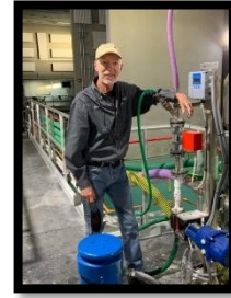
Marc Empson in his last few shifts operating the Water Plant
