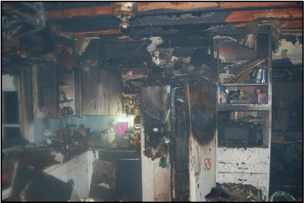
222 21 st Street House Fire
