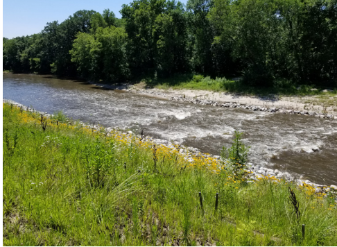
Stream bank improvements implemented on Ioway Creek near Lincoln Way are similar to those being proposed for Brookside Park.
