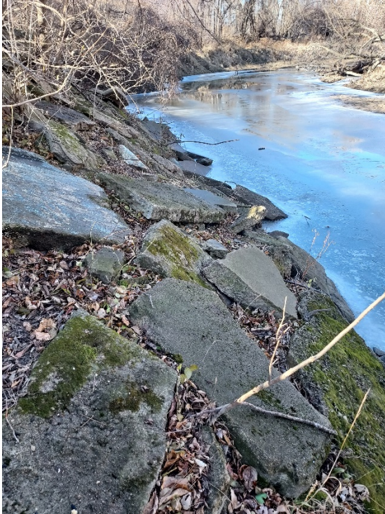
Figure 3. Photo of existing broken-concrete riprap along the right bank of Ioway Creek between stations 6+00 and 7+00.
