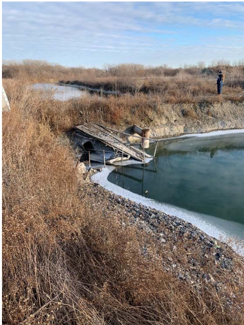
Photo 29: 2019 Pipe structure connecting west channel to northern area in the ash pond.
