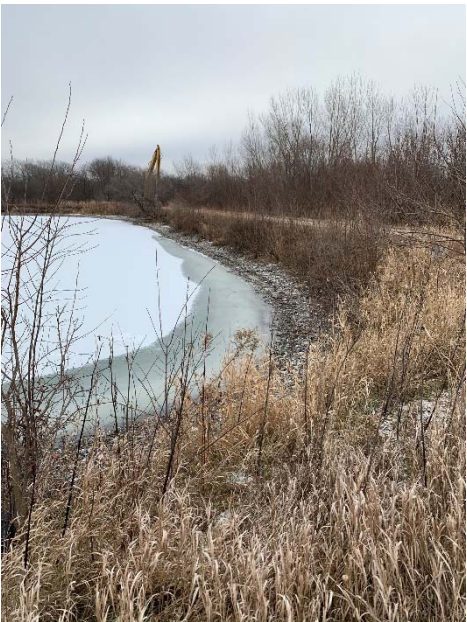
Photo 7: 2019 Erosion along inside slope south embankment
