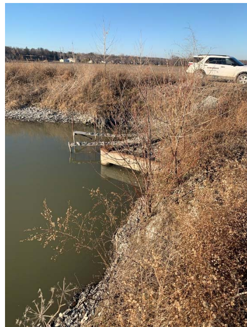
Photo 30: 2020 Pipe structure connecting west channel to northern area in the ash pond.
