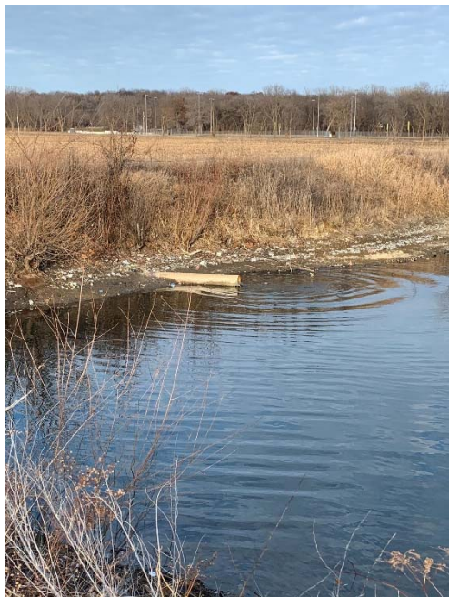
Photo 31: 2019 SEP floor drain and cooling tower blowdown discharge pipe into the north side of north storage area in the ash pond.
