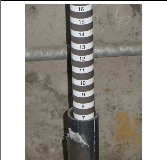
Photo 17: 2019 Gauge located within pump house (CW-2)
