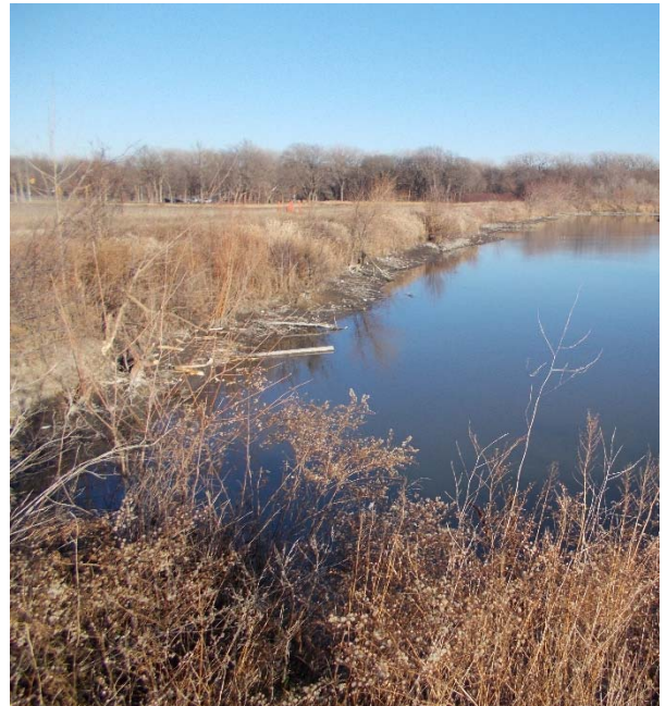
Photo 32: 2020 SEP floor drain and cooling tower blowdown discharge pipe into the north side of north storage area in the ash pond.
