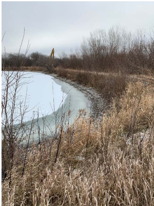
Photo 23: 2019 Erosion on inboard slope southeast portion of the ash pond from south looking northeast. See Area 2 for location.
