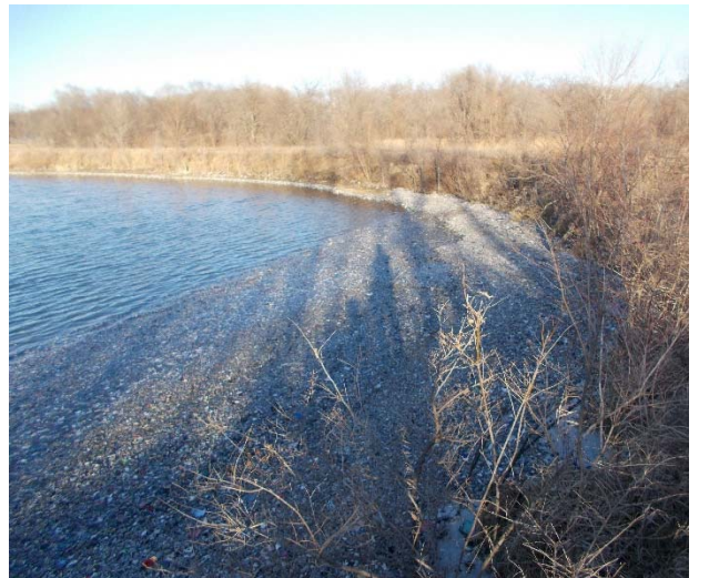
Photo 8: 2020 Erosion along inside slope south embankment
