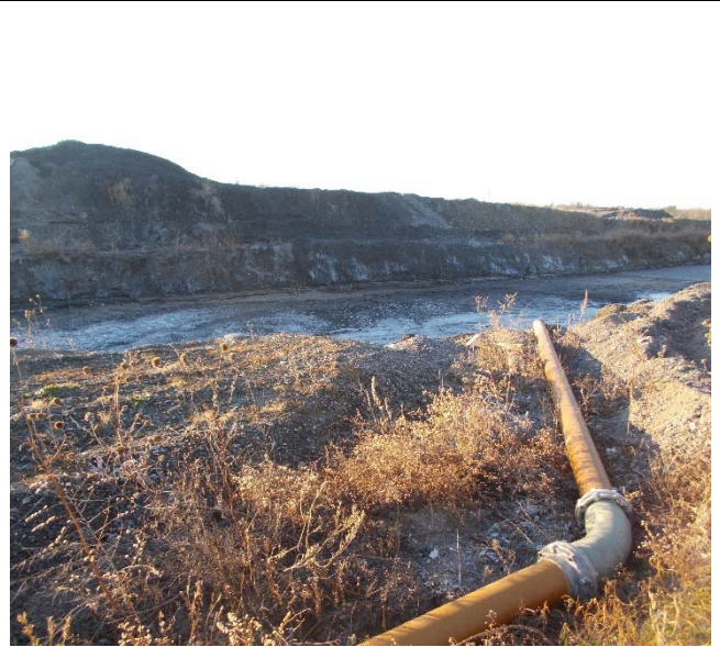
Photo 26: 2020 Ash sluice pipe to West Ash Pond Receiving Ditch
