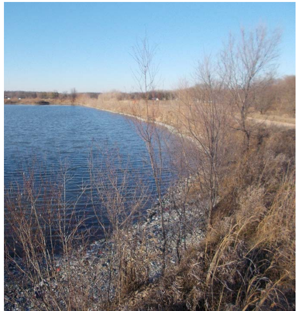
Photo 24: 2020 Erosion on inboard slope southeast portion of the ash pond from west looking along the south/southeast. See Area 2 for location.
