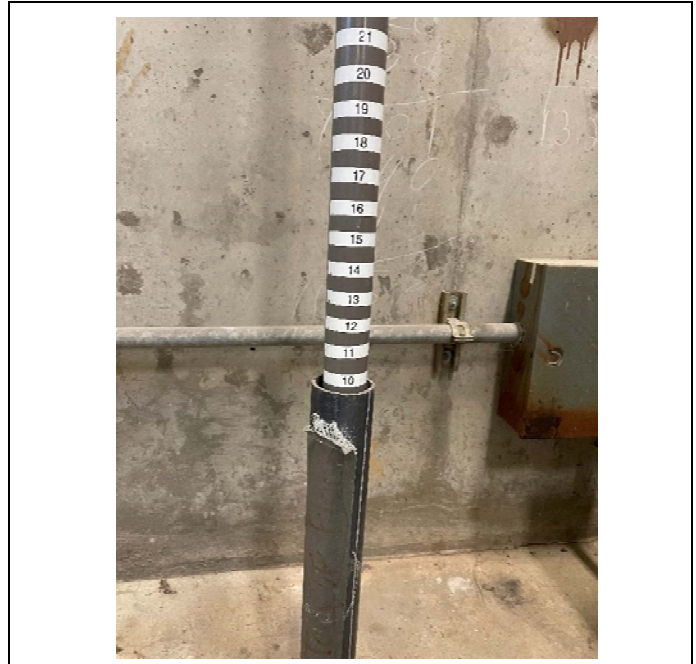
Photo 18: 2020 Gauge located within pump house (CW-2)
