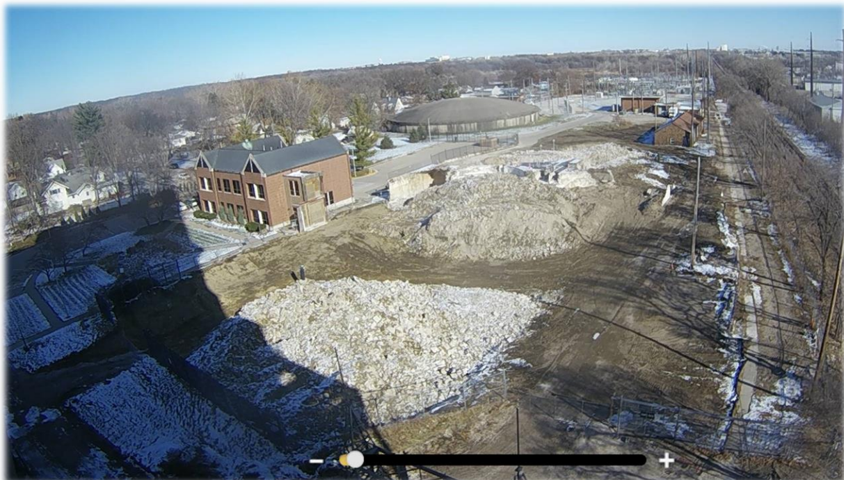
Demolition of the old Water Plant, as seen from the Power Plant
