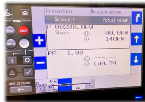
A screen from the methane engine generator (MG) controls showing MG2 being set to operate at 200 kW but only being able to achieve 140 kW.
