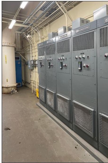
Figure 8.02-19 Influent Pump VFDs and 30-inch Influent Wastewater Pipe
