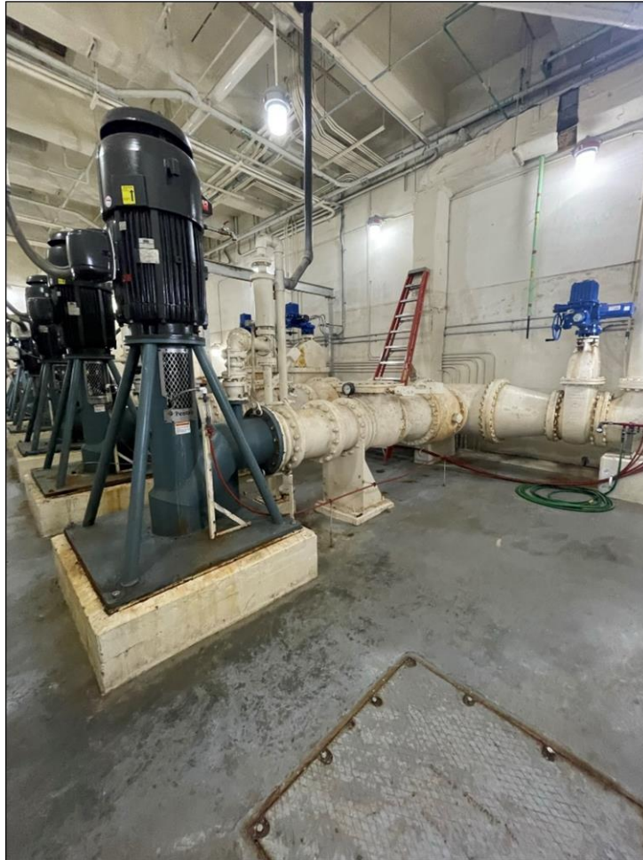
Figure 8.02-6 VTSH Raw and Equalization Pumps
