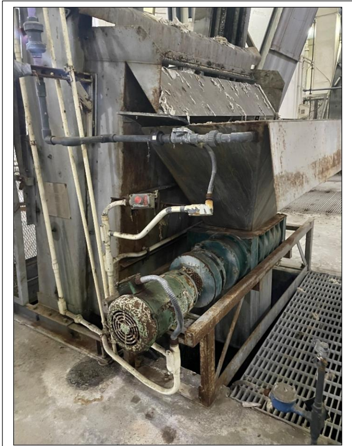
Figure 8.02-2 Original Infilco Degremont Screen and Grinder System
