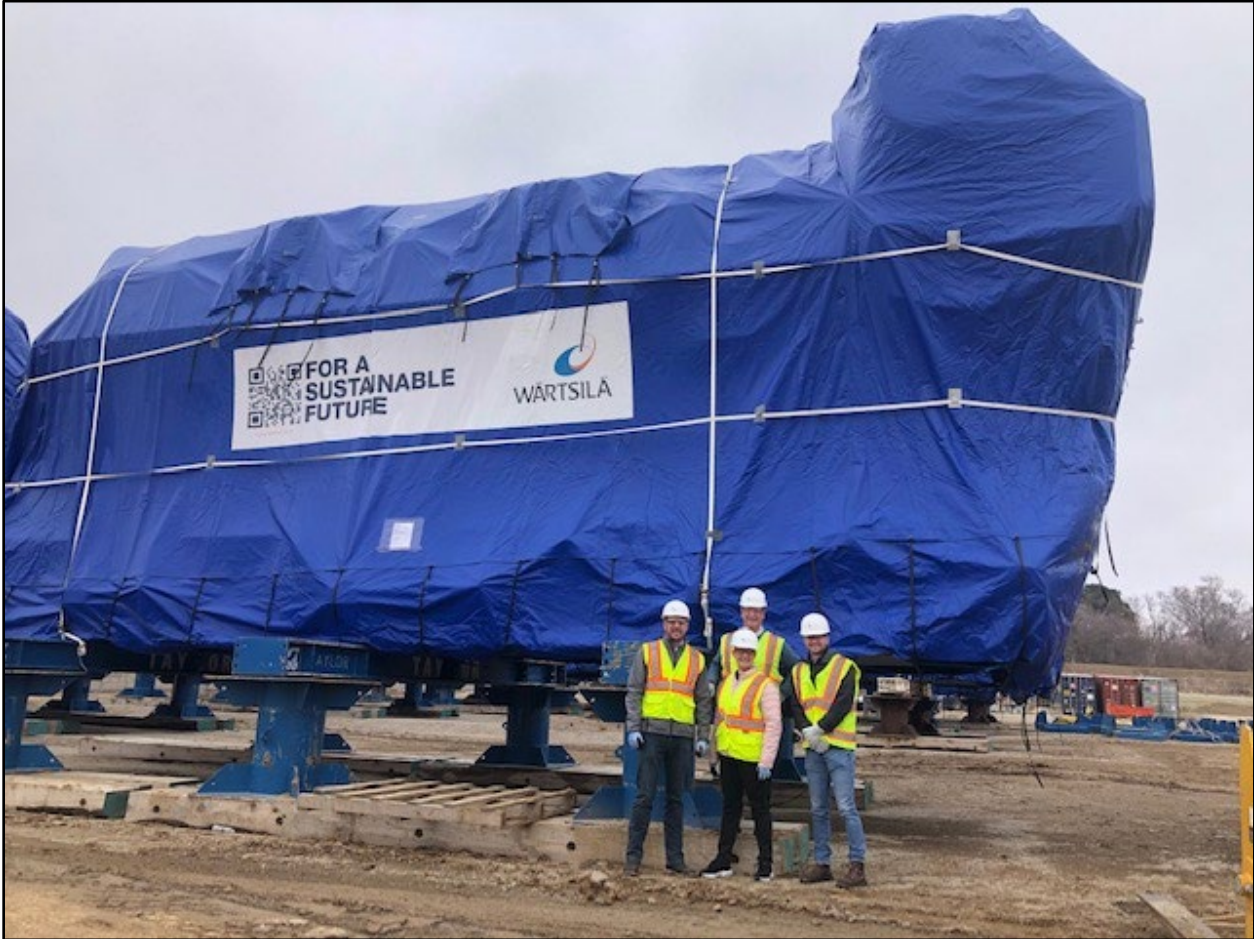
The above picture shows Electric staff standing in front of one of the nine fast-start natural gas Wartsila engines OPPD is installing at one of the new power generation stations being built.
