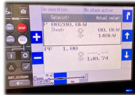
A screen from the methane engine generator (MG) controls showing MG2 being set to operate at 200 kW but only being able to achieve 140 kW.
