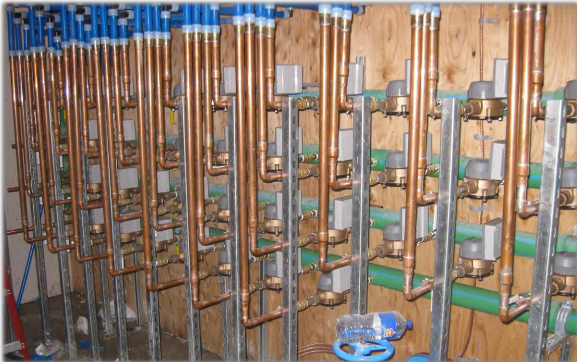
Example of a meter manifold that is typical of a large apartment building.
