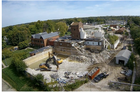
Demolition work at the former Ames Municipal Water Plant includes recycling of debris.
