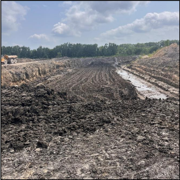
July 24: This photo shows continued work on the separation berm, which was slowed due to wet soil and ash conditions.
