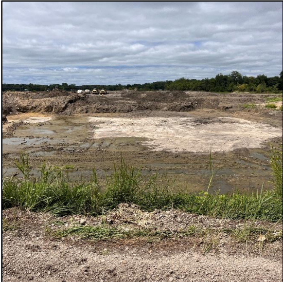
August 6: This photo shows the former pond area looking north. The contractor has excavated most of the ash from the southern part to start the drying process on the northern part.
