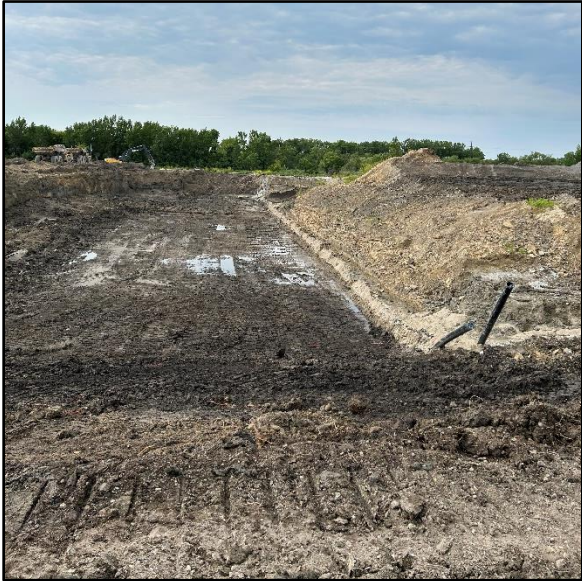
July 17: This photo shows excavation progress toward creating a clay separation berm, which will become the eastern side of the ash closure area.
