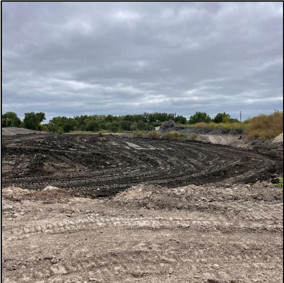
August 8: This photo shows compacted ash in the closure area, which will ultimately be covered with a geomembrane to create the final closure area.
